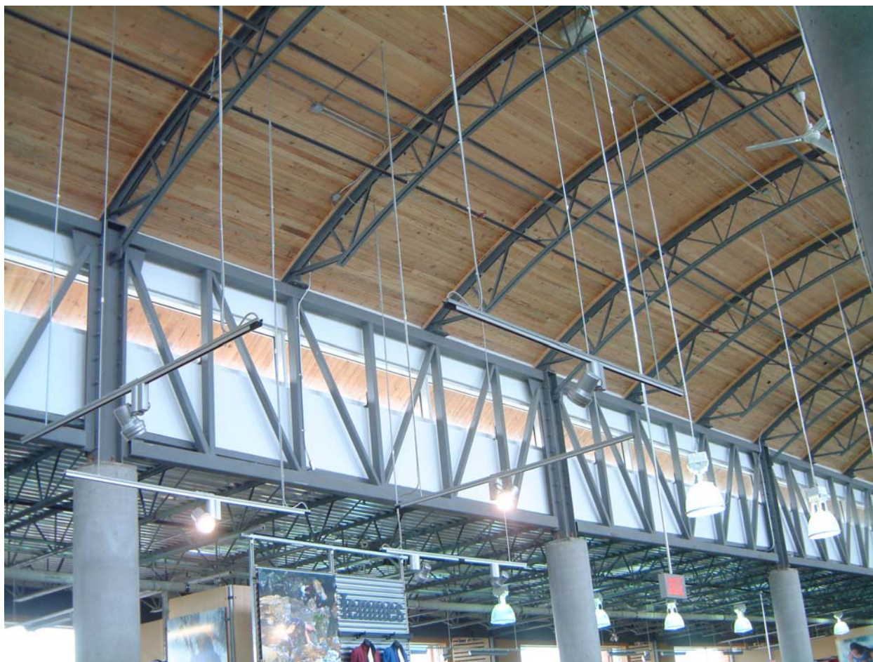
Figure 2 – The main trusses of the Montreal Mountain Equipment Coop include reused HSS
