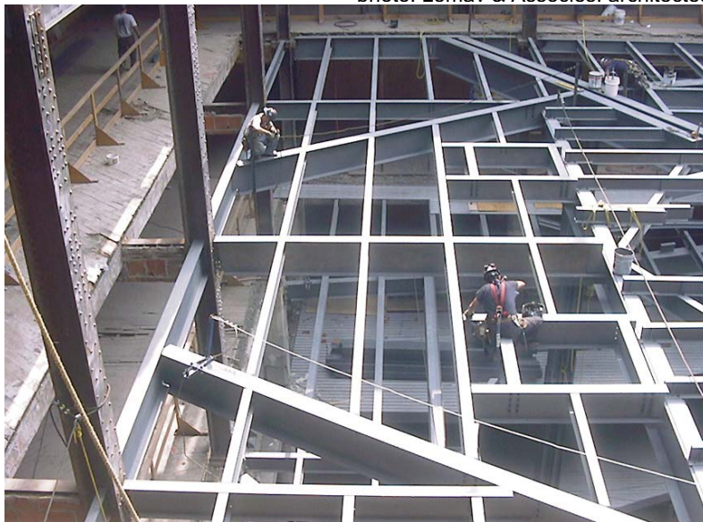
Connecting new beams of the Complexe Les Ailes to old columns of the Eaton Building in Montreal
